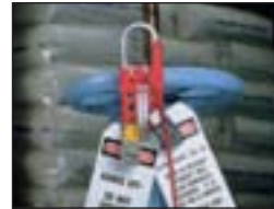
Lockout gate valves
