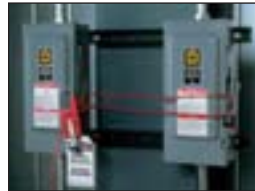
Lockout single or multiple electrical disconnects
